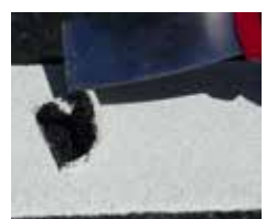
Fig. 4 Perform chisel test to verify bond. Evidence, as shown, of asphalt aggregate bonded to the underside of the lifted material indicates good adhesion.
