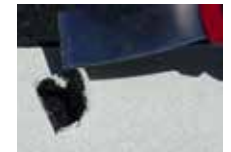
Fig. 8 Perform chisel test to verify bond. Evidence of aggregate bonded to the underside of the lifted material indicates good adhesion.
